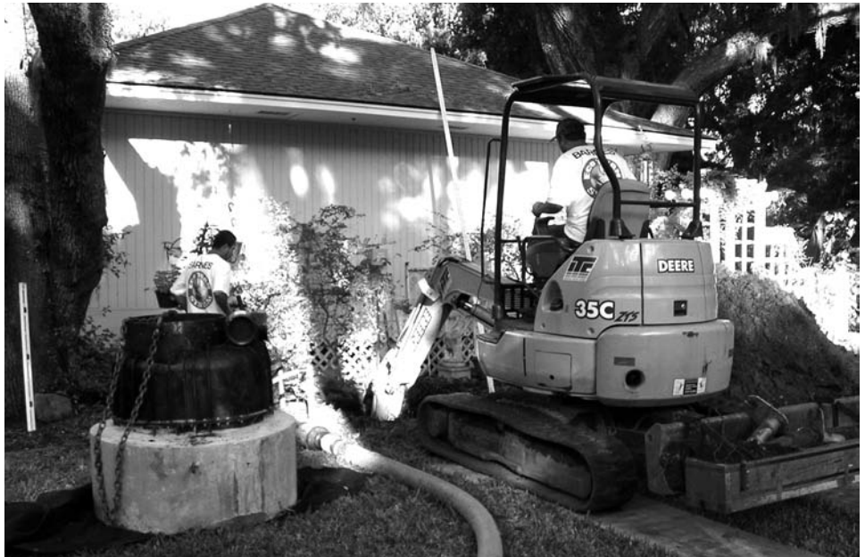
The Oak Marsh neighborhood off Spanish Wells Road was the first to receive a Low-Pressure Sewer system from the PSD. At left is a Low-Pressure Sewer pump unit, which grinds household waste and pumps it into the PSD's public sewer system.
