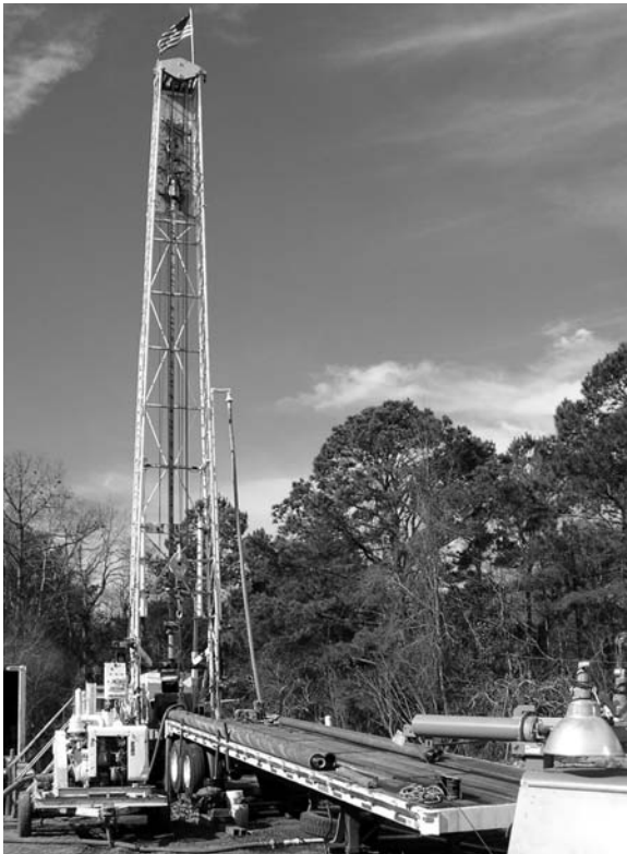
This drill rig was used to drill a test well into the Middle Floridan Aquifer on Jenkins Island, across from Windmill Harbour, as part of the PSD's reverse osmosis drinking water treatment plant project.
