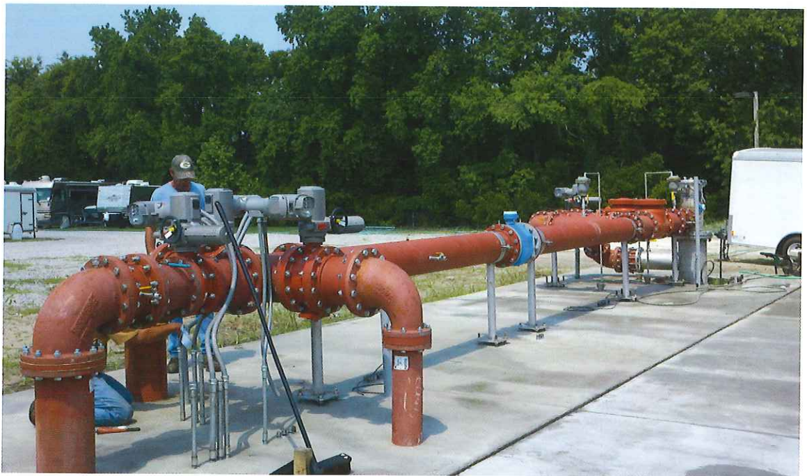
Hilton Head PSD's new Aquifer Storage & Recovery (ASR) well is located off Royal James Drive in Hilton Head Plantation. The well stores treated drinking water during the winter months of low demand and withdraws it for re-treatment and distribution during the summer months of high demand. This is Hilton Head Island's first-ever ASR well. It is needed in order to ensure a long-term and high-quality supply of drinking water in the face of ongoing saltwater intrusion into the island's traditional groundwater source.
