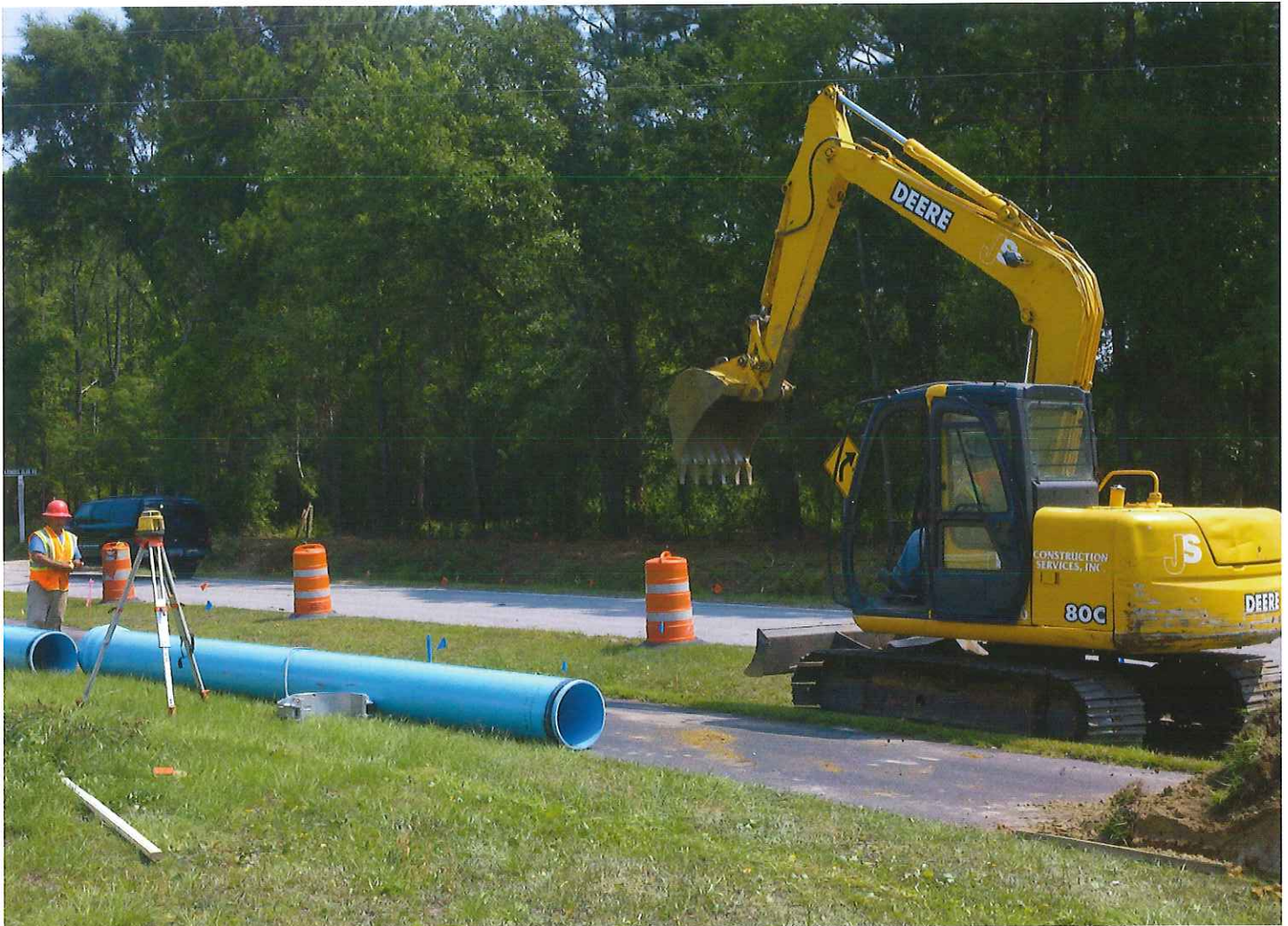
The PSD is installing a water transmission main in the Wildhorse and Gumtree roads area as part of a water supply project to combat the effects of saltwater intrusion in our traditional groundwater source.
