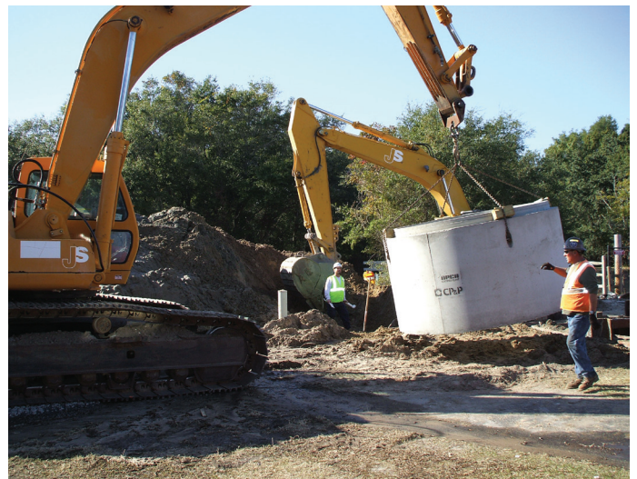
Construction workers install concrete for the PSD's new sewer pump station that will serve the Baygall neighborhood.
