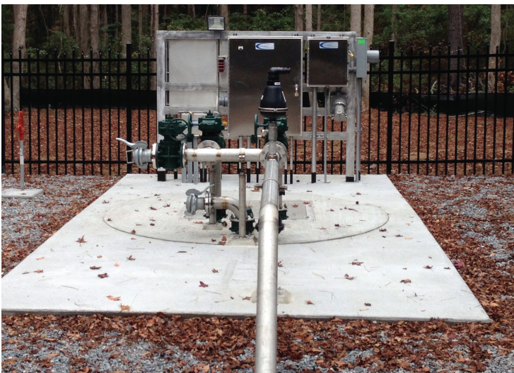
The PSD's new sewer pump station near the Spanish Wells Business Center brings sewer service to the mid-Spanish Wells Road area, including Bluebell Lane. The project included sewer line installation and was jointly funded by the Town of Hilton Head Island.
