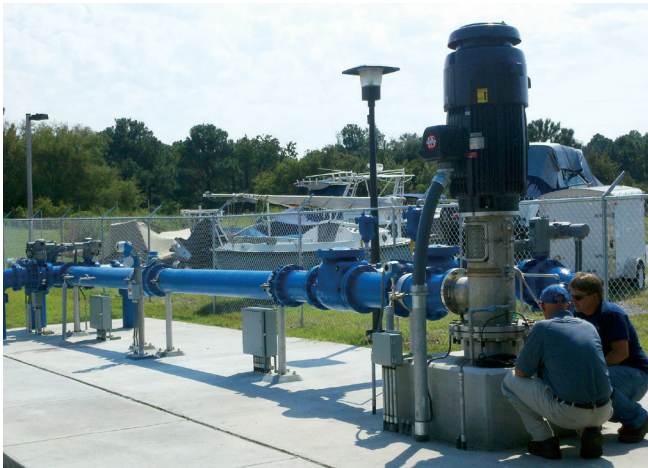
The PSD built the island's first-ever Aquifer Storage & Recovery (ASR) well in 2011. It is located inside Hilton Head Plantation.
