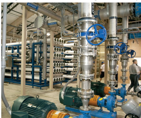
The interior of the PSD's RO Plant.
